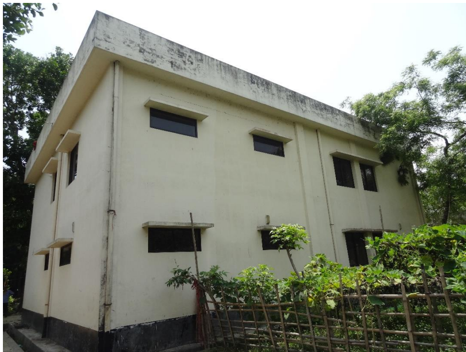
Figure 6.12: Backside Building Condition
