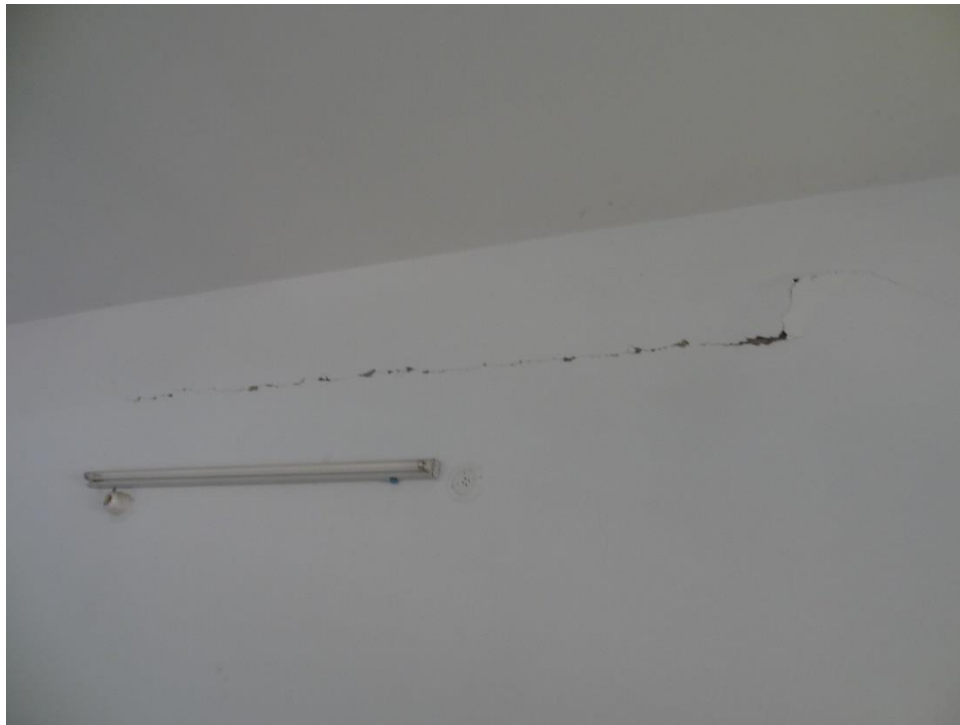
Figure 6.1: Cracked Plaster in between beam & wall joint
