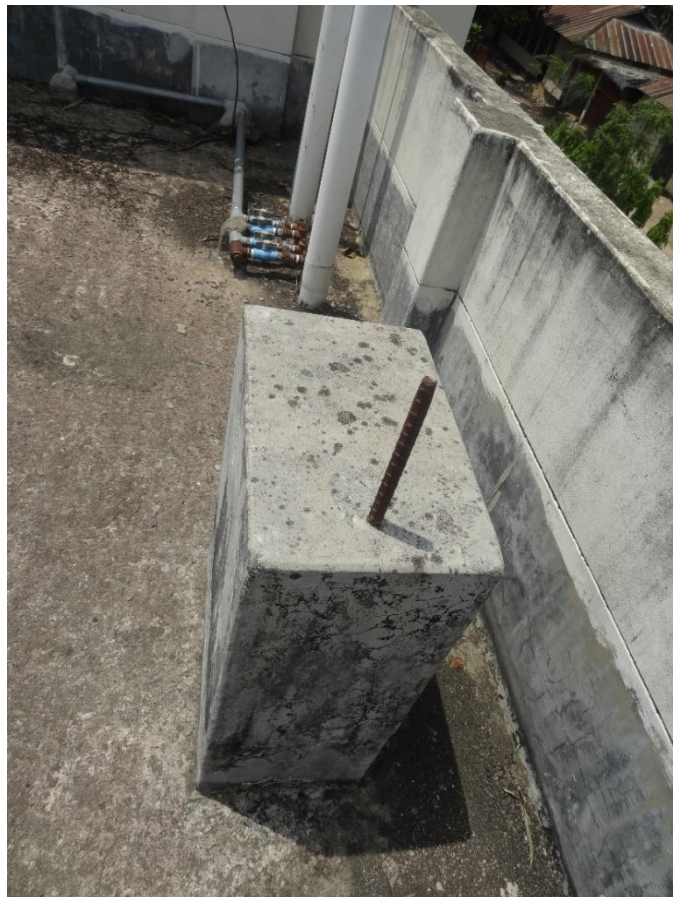
Figure 6.4: Exposed Rebar of Roof False Column
