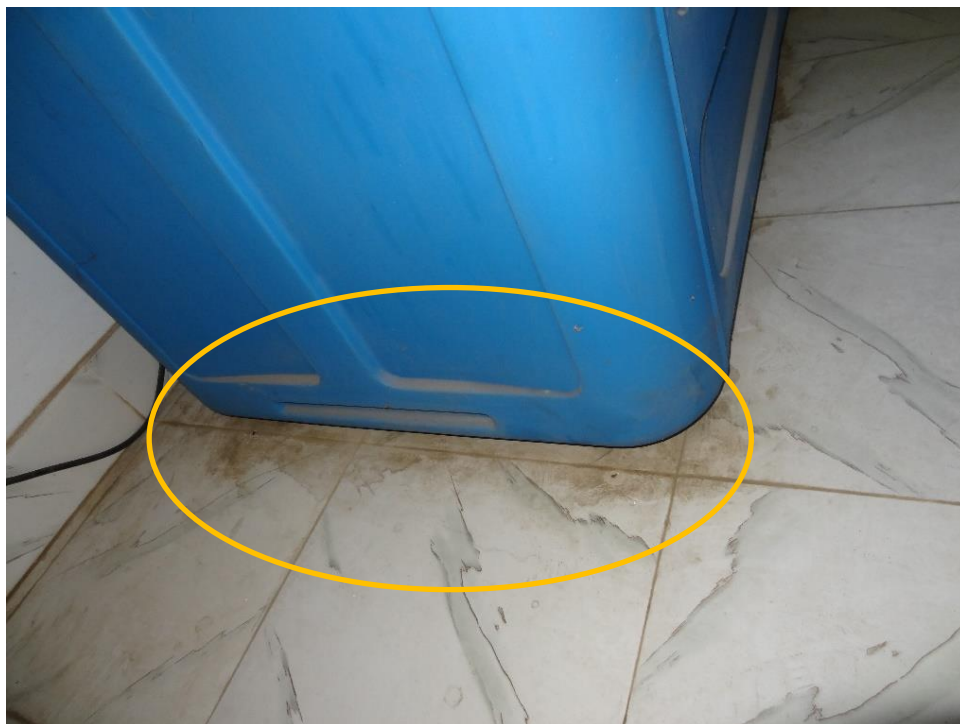
Figure 6.10: Sign of past water mark during rainy season at Ground Floor
