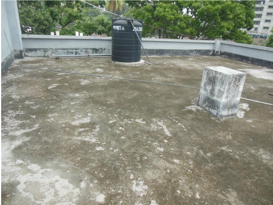
Figure 6.1: Trace of Water Logging and Roof Dampness
