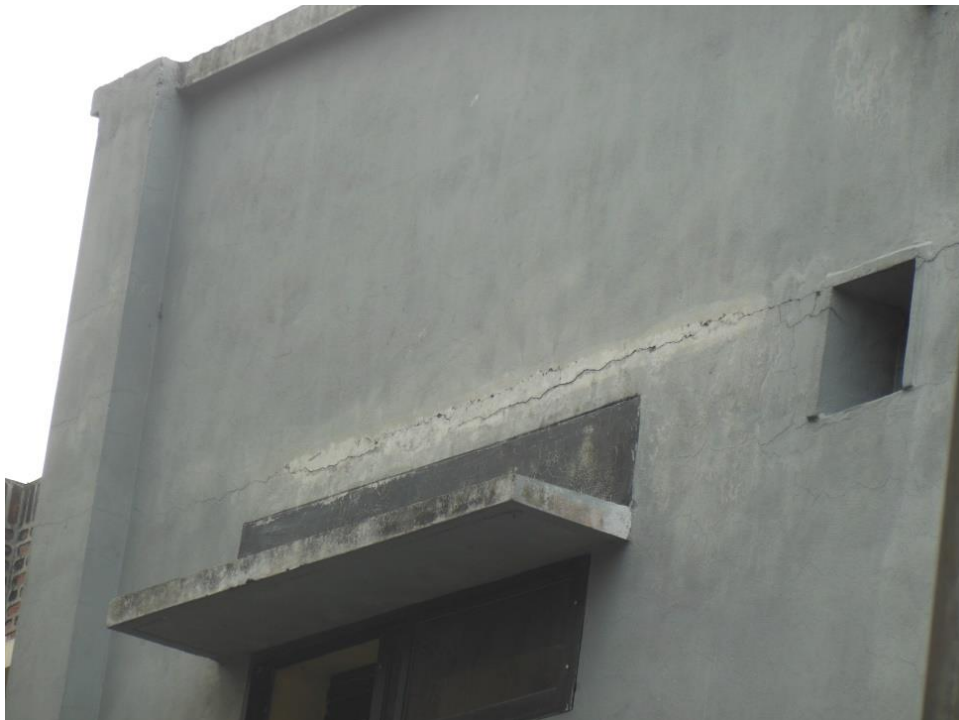
Figure 6.2: Minor Cracks Found On the Exterior Partition Wall
