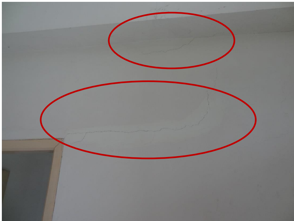
Figure 6.1: Cracked Partition Wall Plaster
