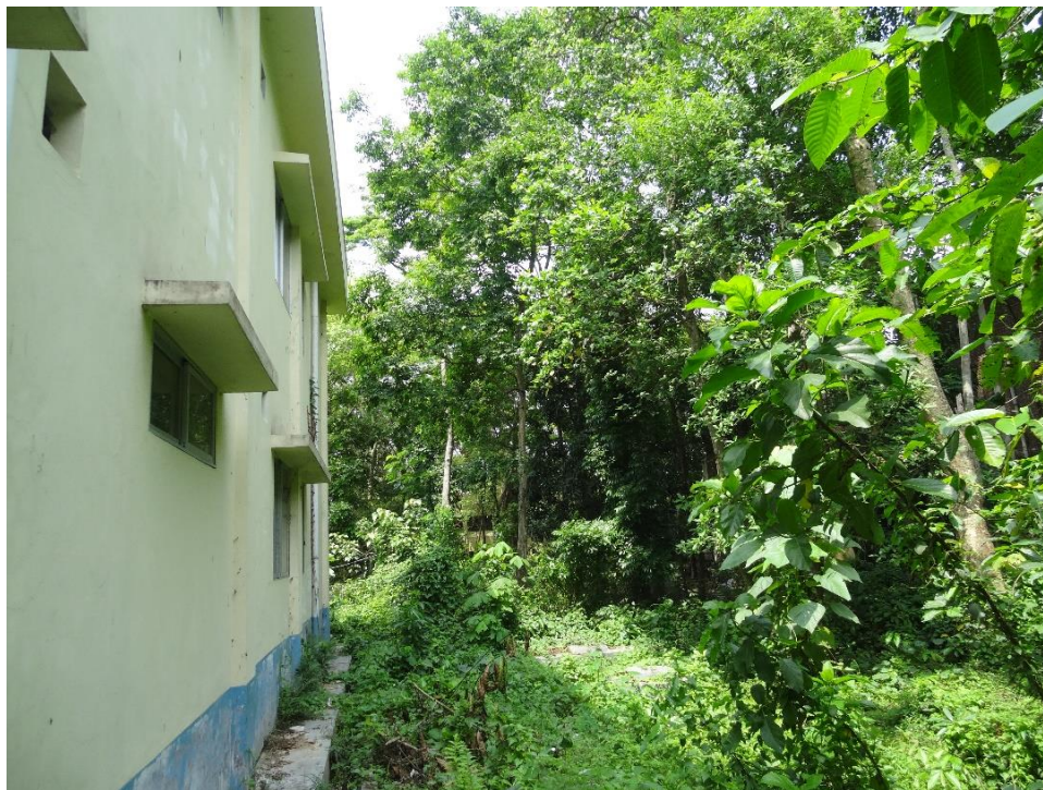
Figure 6.13: Backside Building Condition
