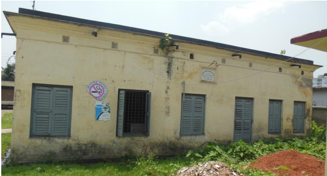
Figure 6.4: Back side condition of building
