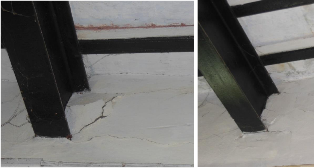
Figure 6.1: Cracks in load bearing wall below steel beam
