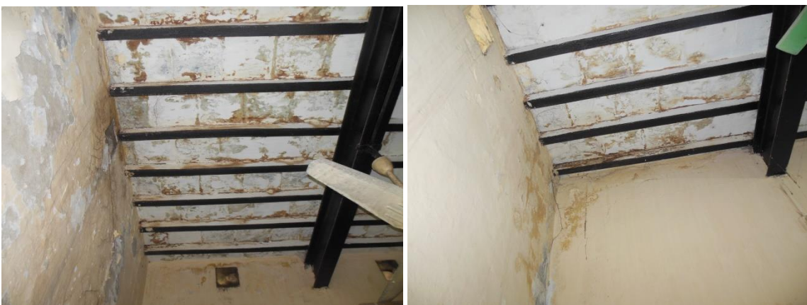
Figure 6.3: Dampness in roof slab
