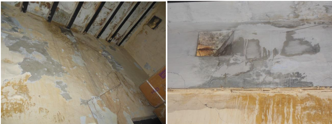
Figure 6.2: Dampness in load bearing wall
