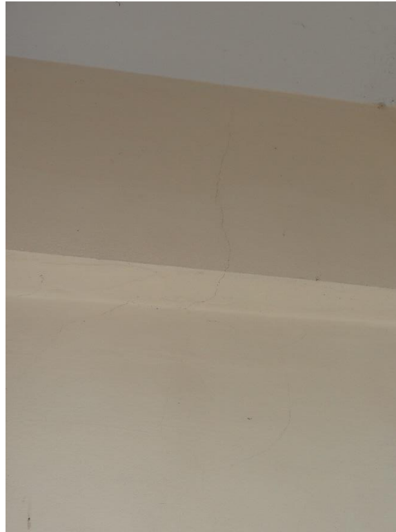
Figure 6.7: Visible minor cracks in the plaster of beam (1 st floor)
