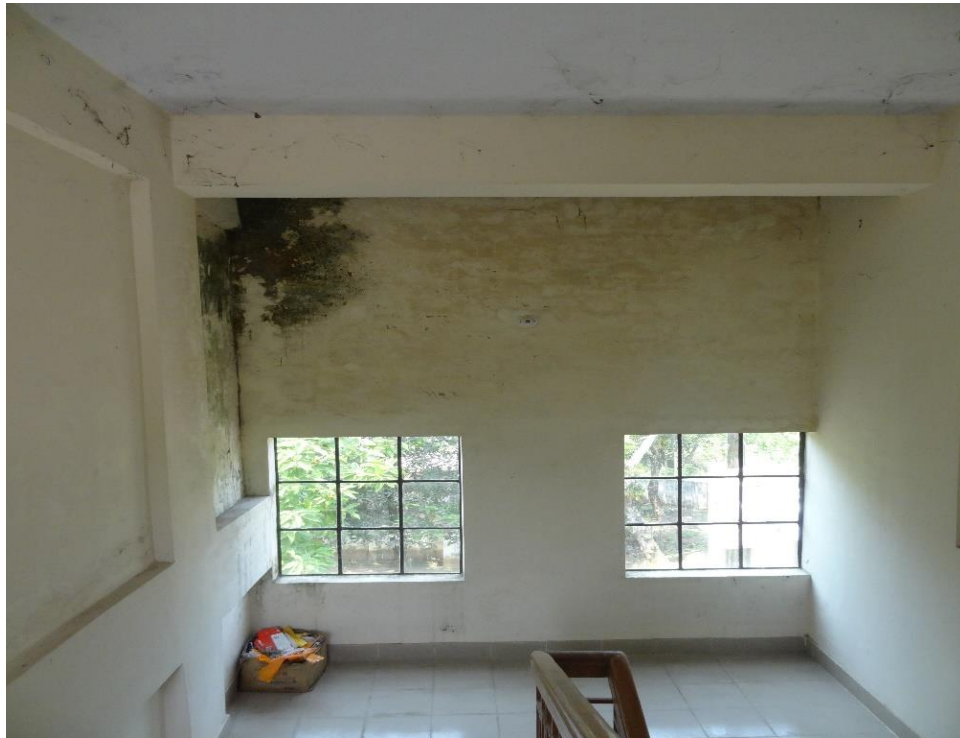
Figure 6.1: Partitions wall affected by moss at stair landing Portion
