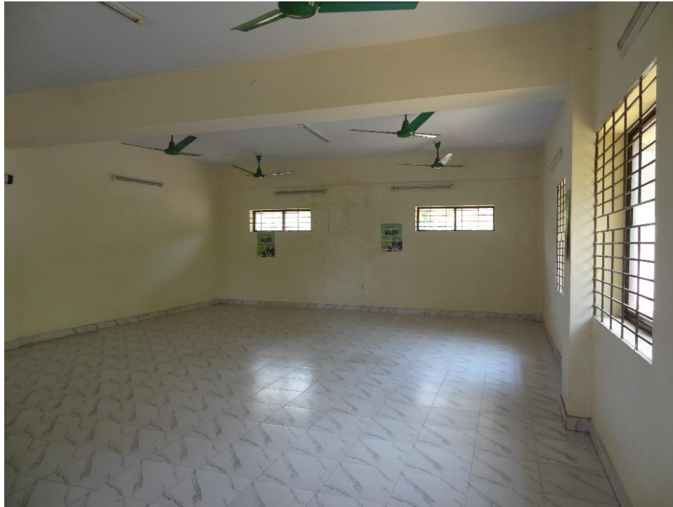
Figure 6.5: Existing Conference Room with dampness in side wall at 1st Floor
