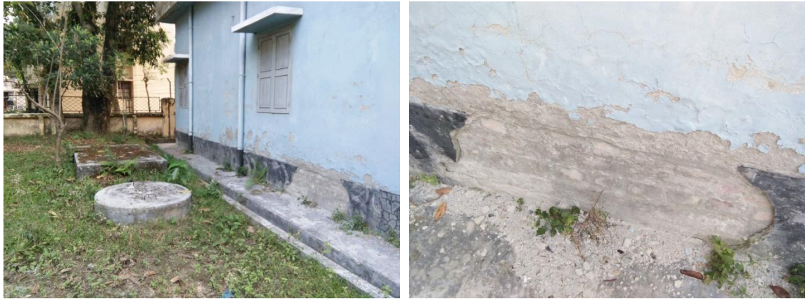
Figure 6.3: Damaged outside plaster
