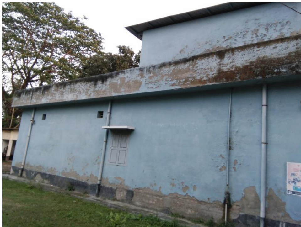
Figure 6.6: Outside paint condition
