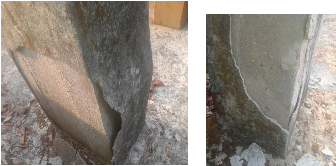
Figure 6.4: Damaged on column plaster
