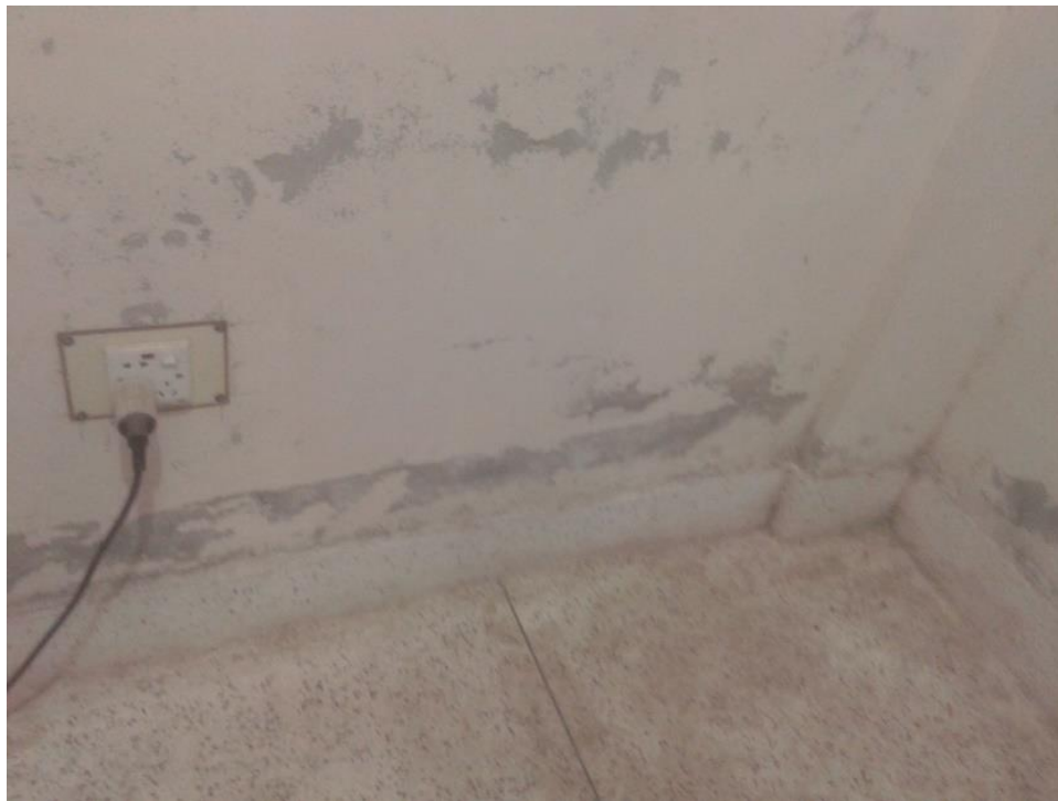
Figure 6.7: Dampness in interior wall of cold storage room
