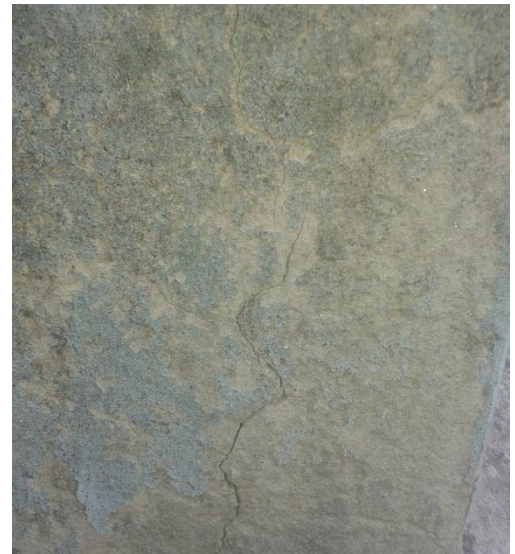
Figure 6.1: Crack in Column
