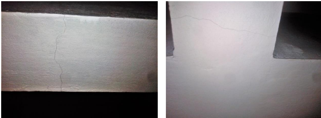
Figure 6.8: Crack in Waffle beam in cold storage room
